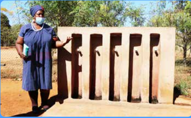
Above: The water saving taps that the school installed to conserve water.
