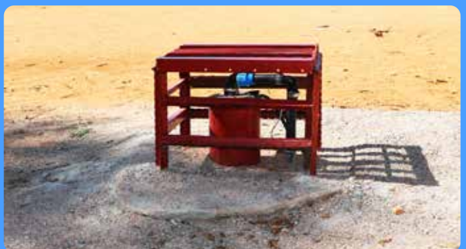
Above: The 90m deep borehole that supplies Ramaahlo Primary School with water.
