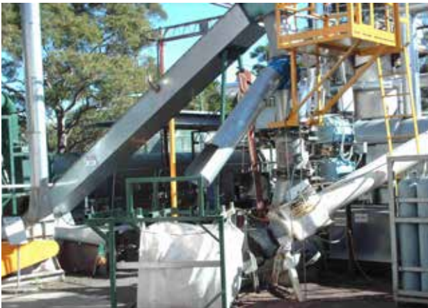
(iii) A commercial biochar plant in Australia. (Source: http://www.biorenewal.org/home/biochar-production-technology )
