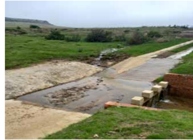
Above: A rehabilitation structure consisting of the multiple types of interventions in one such as a: Brick weir, Concrete road crossing, Concrete strips and Stone masonry.
