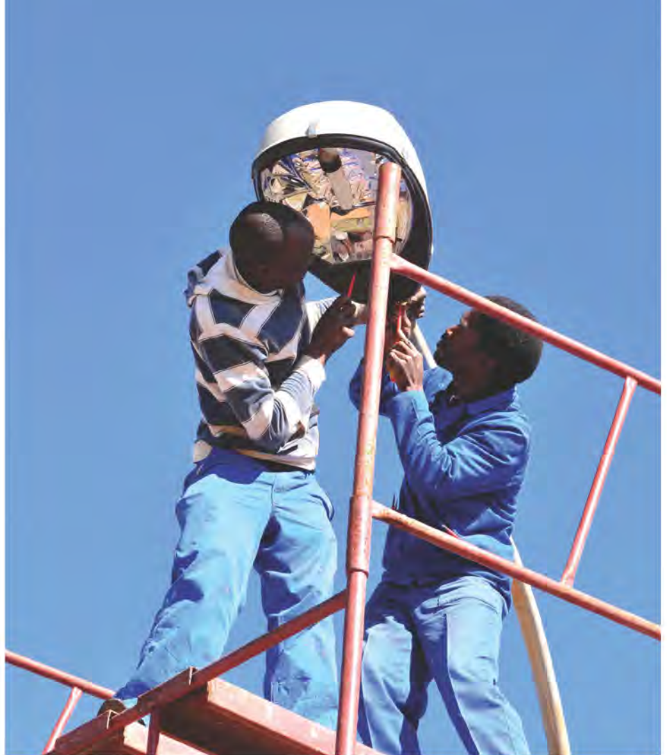
A team installing energy efficient floodlighting at one of the official training venues.
