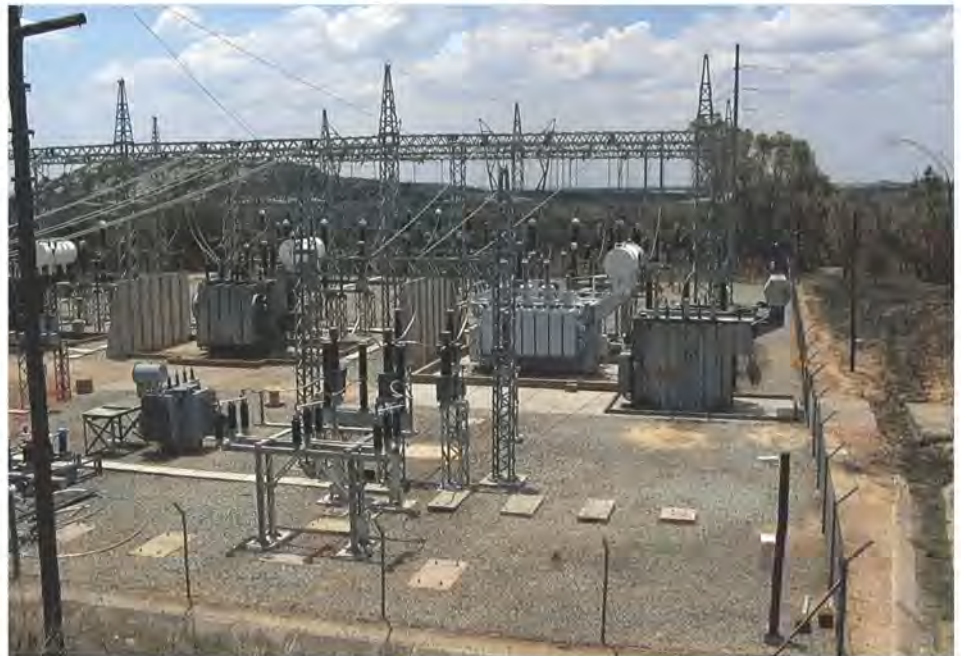
The Silica Substation in Polokwane was among the many electrical infrastructure upgrades in South Africa necessary to host the 2010 event
