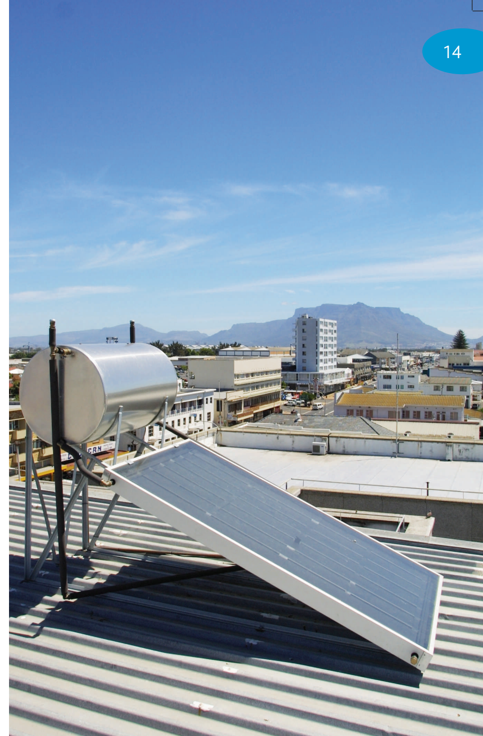
Solar water heating
