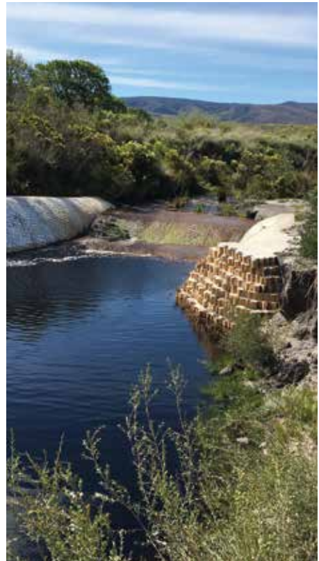
Above: A chute-drop was constructed from geo-cells and concrete to prevent further erosion of the Pietersielieskloof wetland system.
