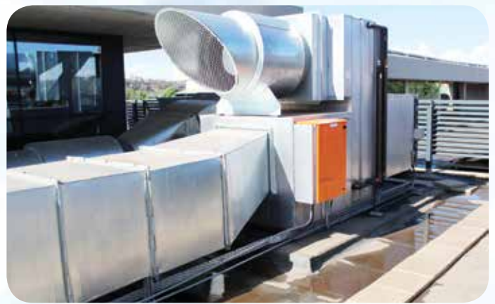
Above: The building has a rainwater harvesting system, water-wise indigenous plants and efficient irrigation systems.
