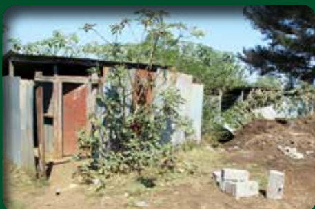
Above: the old toilet structure that was being utilised by the schools learners and teachers before the new toilet was built.
