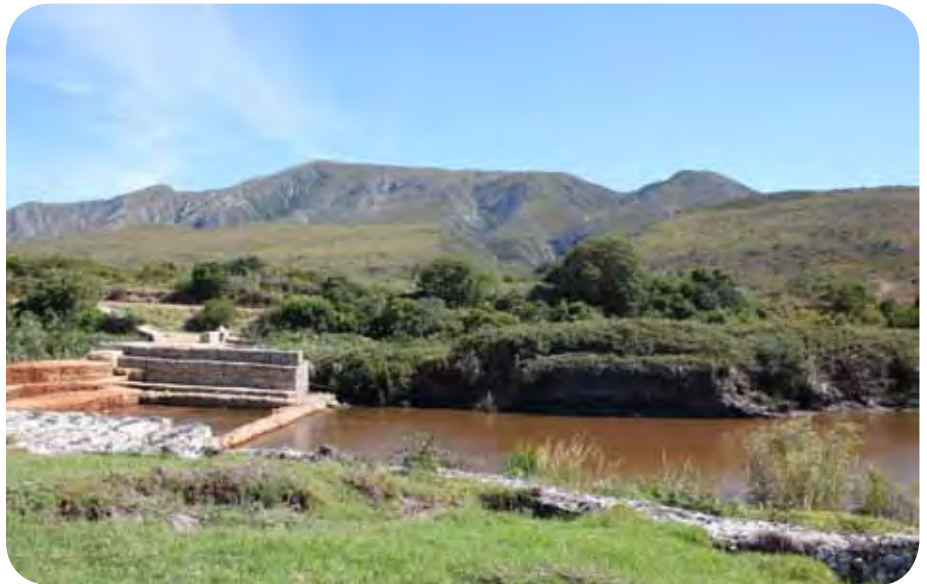
Over the past 11 years, 11 large gabions and concrete structures have been built at a total cost of over R10 million, to combat erosion that threatened the remaining large, intact wetlands. It is estimated that this work has improved water availability by approximately 32 000 litres of water per day per hectare cleared.
