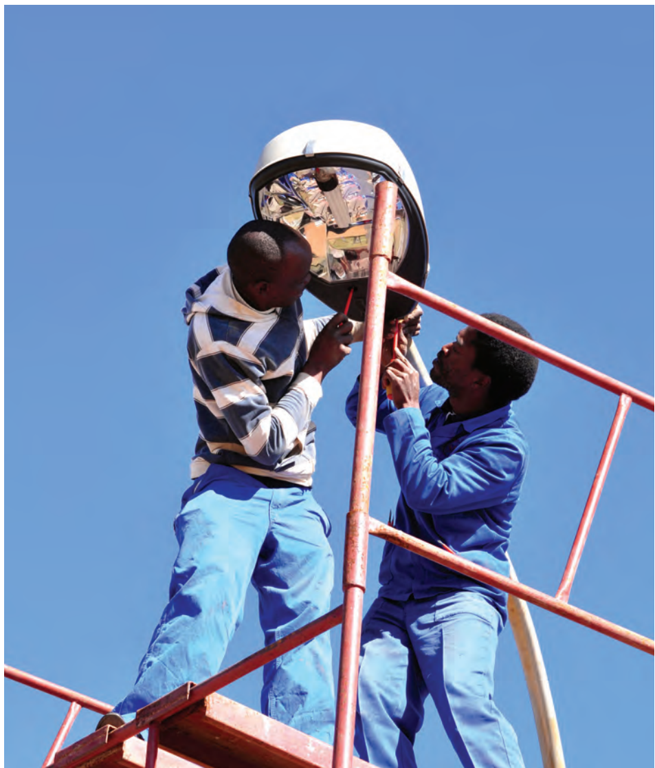
A team installing energy efficient floodlighting at one of the official training venues.
