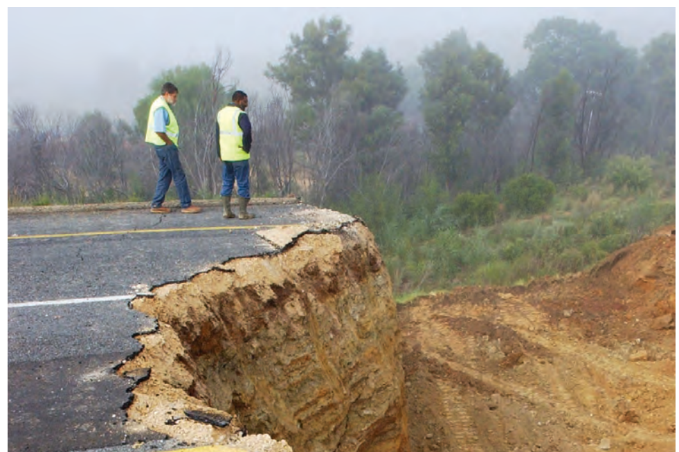
N2 highway destroyed by floods. Photography: Trace Images / Brenton Geach
