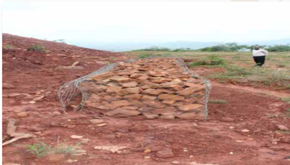
Picture 3: Hilltop 01 with a gabion placed thereon by the offenders in an attempt to prevent or minimise the soil erosion.
