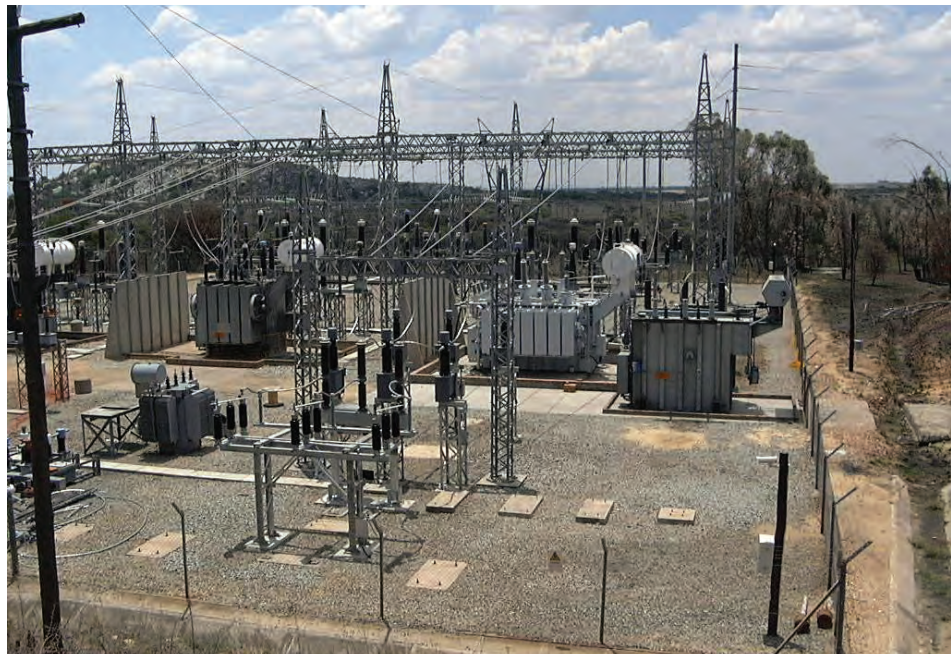
The Silica Substation in Polokwane was among the many electrical infrastructure upgrades in South Africa necessary to host the 2010 event
