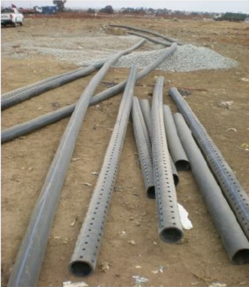
7. Perforated well pipes
